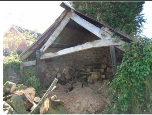
Photo 28. Lodway Farm Building LF6 – the wood store is a simple structure with no bat roost potential. Date: October 2018
